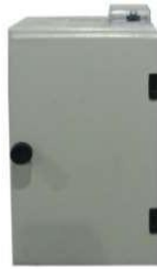
Gambar 2. 16 Box Control Panel (Sumber: Rahmad Riyanto, 2017)
