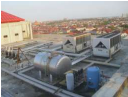
Gambar 2.2. Instalasi sistem tata udara Chiller Air Cooled Single Screw
