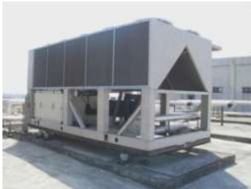
Gambar 2.3 Chiller (unit pendingin)
