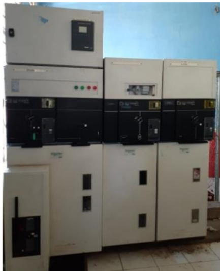
Gambar 5. Panel Kubikel 20kV
