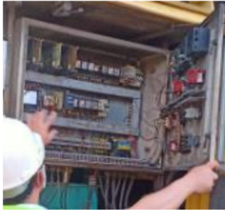
Gambar 4. Panel Control Engine Room
