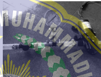
Gambar 3.25 Valve, Pressure Gauge, Pompa
