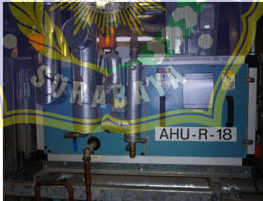
Gambar 2.7 Air Handling Unit
