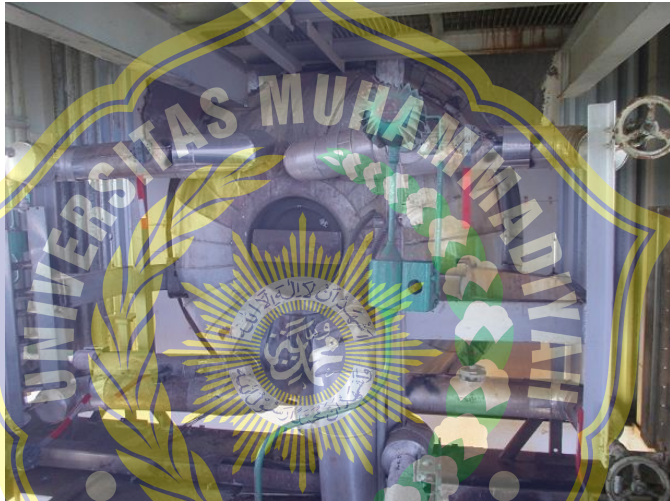
Gambar 2.7 Boiler Drum (Sumber : PLTU 3 Jawa Timur Tanjung Awar-Awar)
