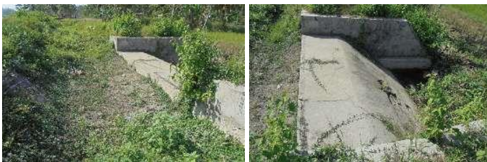
Gambar 4. 10 Bangunan Pelimpah Samping (B.BN.1f) Sumber : Hasil Penelusuran Jaringan Irigasi, 2020
