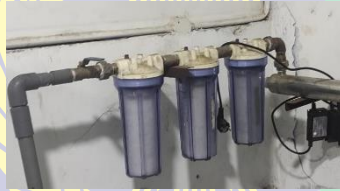
Gambar 4. 3 Filter Air (Sumber: PT. UMSurya Bina Bangsa)
