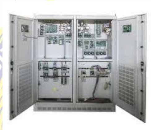
Gambar 2. 3Uninterruptible Power Supply (UPS) (Safi'i, 2023)
