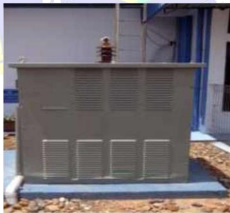
Gambar 2.4. Neutral Grounding Resistance [6]
