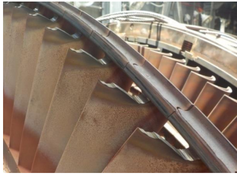
Figure 11. Turbine Stage 2 Bucket Damage before MI CTG 101
