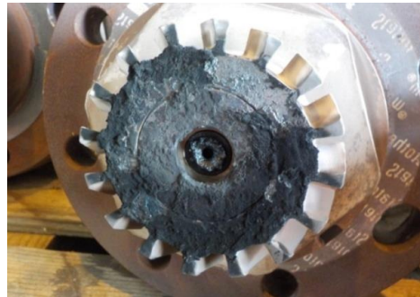
Figure 13. Fouling Conditions on the Fuel Nozzle Before MI CTG 101
