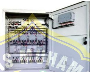
Gambar 2. 13 Panel Distribusi DC
