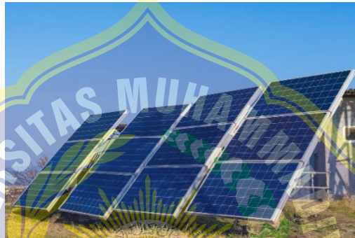
Gambar 2. 1 Solar Panel Array
