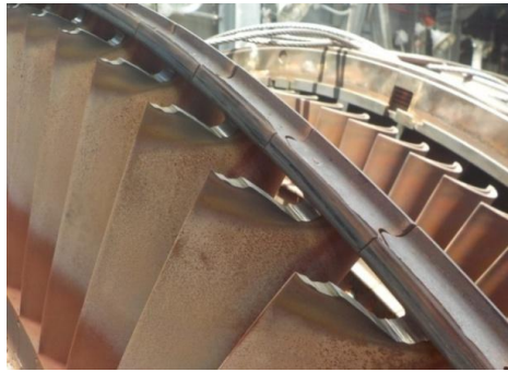
Figure 11. Turbine Stage 2 Bucket Damage before MI CTG 101
