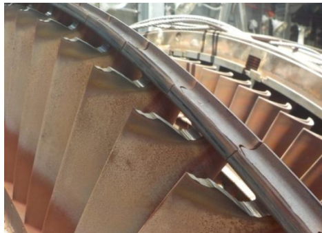
Figure 11. Turbine Stage 2 Bucket Damage before MI CTG 101
